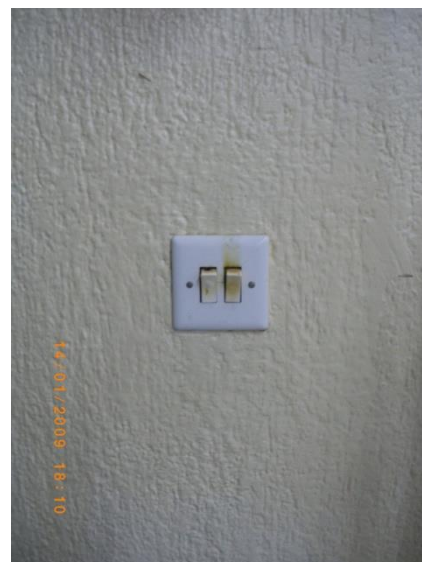
Detalle de interruptor defectuoso
